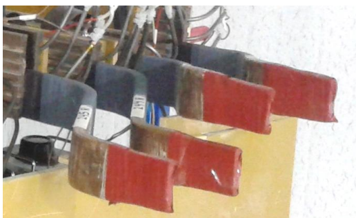
Fig. 2: Generator bars located between hot surfaces
